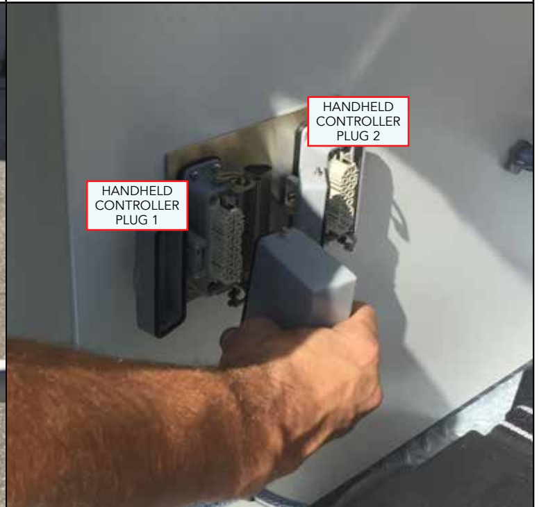
Outside Control Box (back) and Elements
